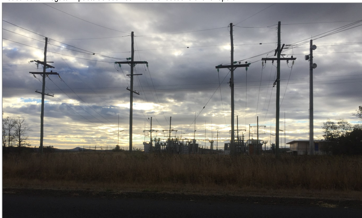
Figure 15 – Ergon Electricity Sub Station as viewed from Yarranlea Road Source: Site Visit, June 2016
