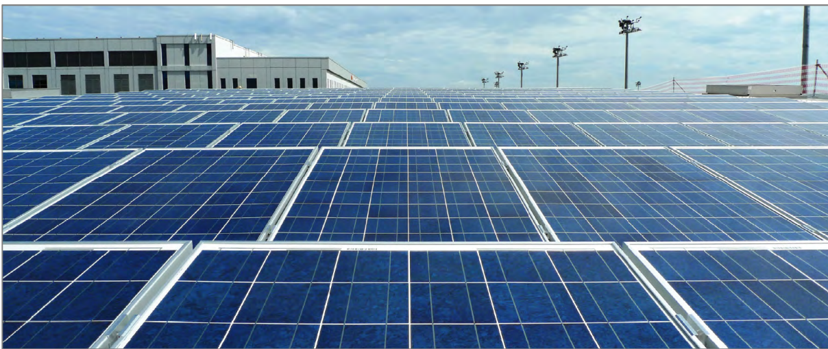
Figure 28 – Solar panels on roof of Changi Airport Budget Terminal, Singapore, 2010 Source: Solar Choice, www.solarchoice.net.au/blog/solar-panels-near-airports-glare-issue , 2013
